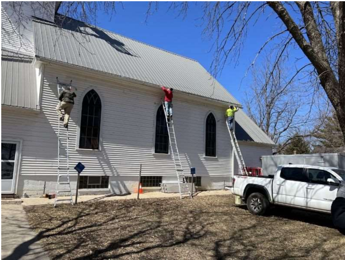
A wall got framed and put up in the basement, a ton of landscaping rock got transplanted to the driveway to keep cars from sinking in, and gutters were put up.
